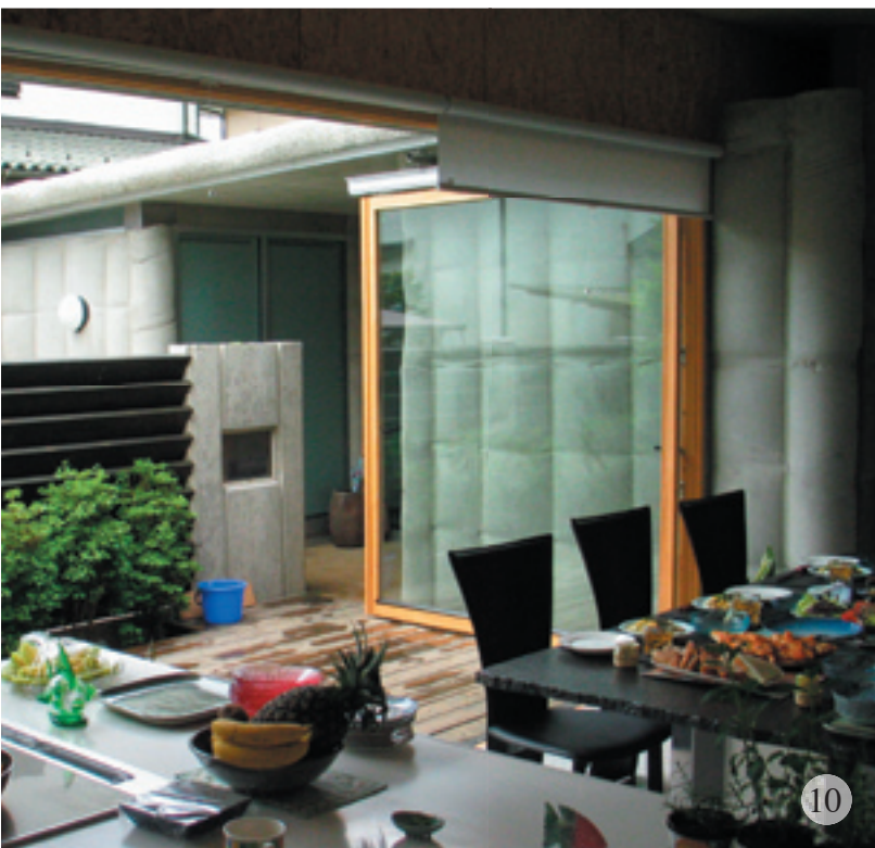
A flexible formwork membrane produces architectural and sculptural forms and surface textures as a direct result of construction decisions and details. The mold surface subtly changes its shape in response to the forces it resists.
