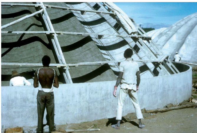
Fig. 9. A Cyprus bin under construction in Nakuru, Kenya (photo by Grant Maslen). Reproduced by permission of Hilary Hann
