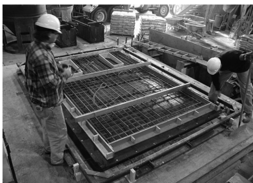
Figure 8. Securing fabric and placing reinforcement in full-scale wall panel formwork (C.A.S.T. photo).
