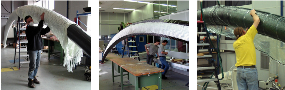
Figures 13-15: Production of the conical arch, by using the vacuum injection method. Both glass and carbon fibres are applied (photos: Rep-air Composites).
