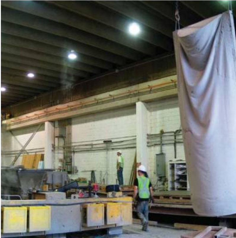
Fig. 46. Thin-shell panel cast from a sheet of hanging geotextile fabric used as...
